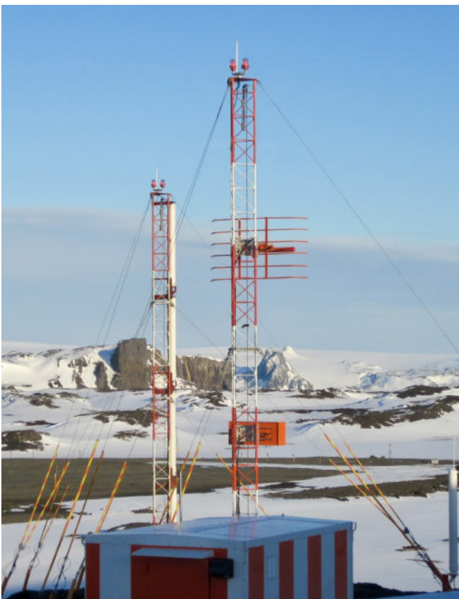
TLS electronics shelter, elevation sensor and uplink antennas
